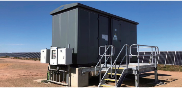
Australia | 1074 Copper Coast Highway 5.9MW Ground Solar Power Plant
