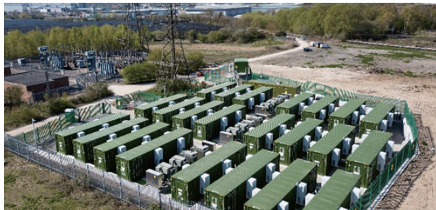
UK | 159MW BESS Project
