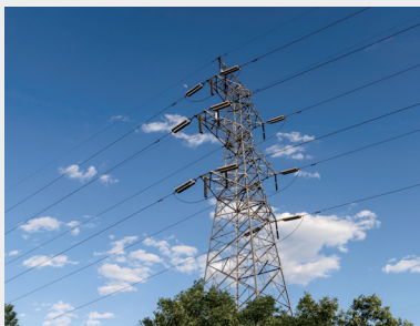
High Voltage Transmission and Transformation
