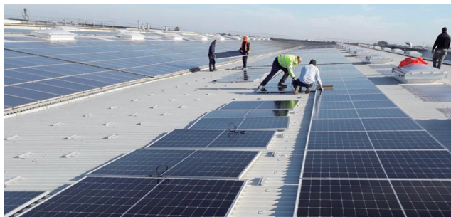
Italy | CARTON PACK S.p.a. 2MW Rooftop Solar Plant
