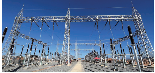
Philippines | Cayanga Bugallon 75MW Solar Power Plant
