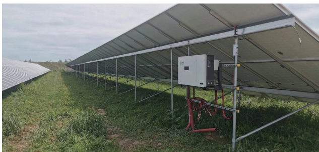
Slovenia | 6MW Ground PV EPC Project
