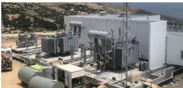
Greece | HEDNO 150kV Transformer Framework Project
