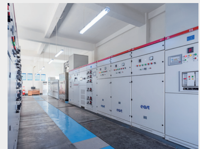
Low Voltage Distribution
