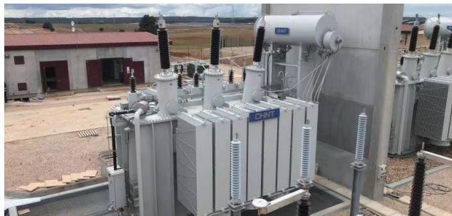
Greece | Terna Wind Farm 150kV Power Transformer Project
