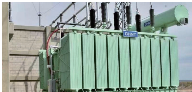
Mexico | Puerto Penasc 158MW+12MW/24MWh BESS Project
