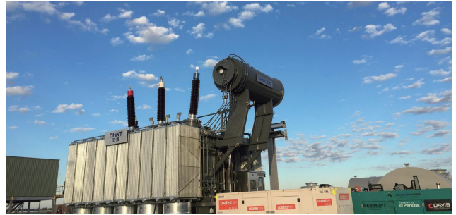
Australia | Nevertie Solar Power Plant
