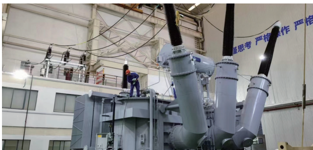
Greece | METON New Energy Power Station Transformer Project
