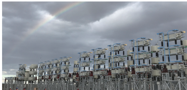
Mexico | Amistad I-IV Station, Magdalena Station and Dolores Station Power Quality Project
