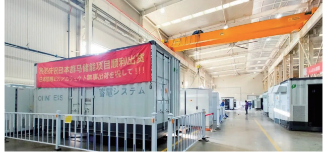
Japan | 500kW/2MWh BESS Project
