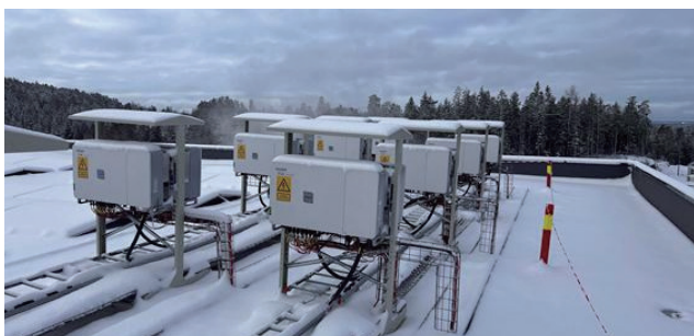
Norway | 2MW Rooftop Project
