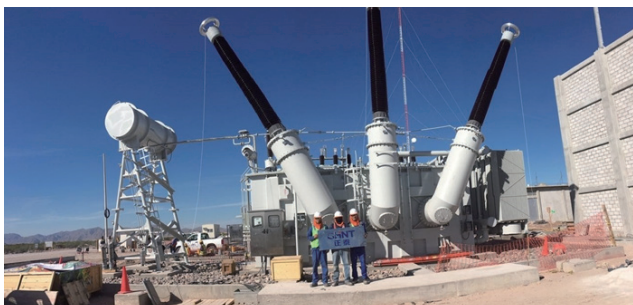
Mexico | Villanueva III Solar Power Plant
