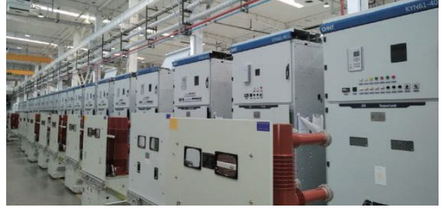
Kazakhstan | Shokpar 109MW Wind Farm
