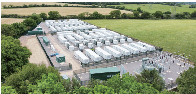
UK | Minety 99.8MW/98MWh BESS Project
